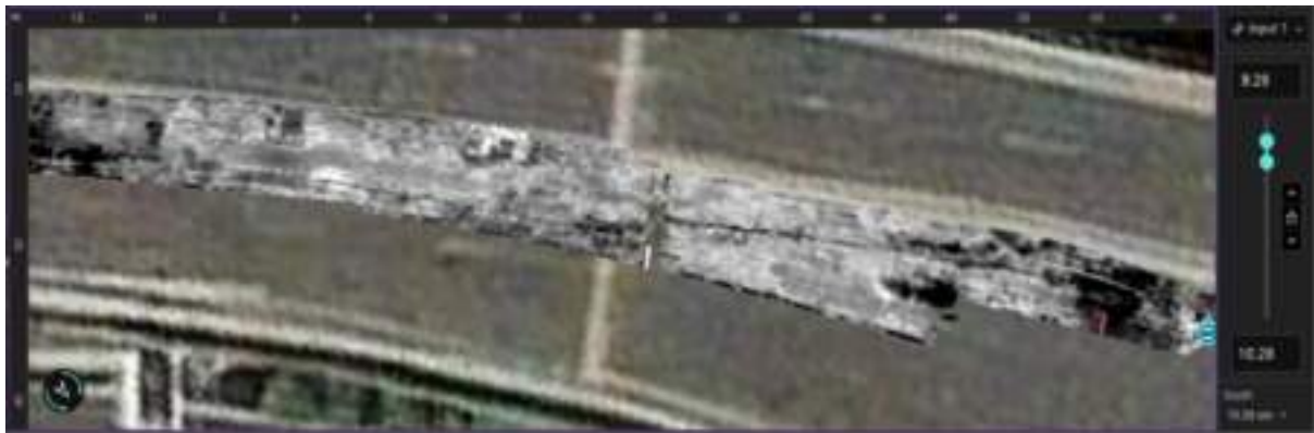
Figure 7. Interface defects between Asphalt-to-Concrete (A/C) layers (Delamination.)
