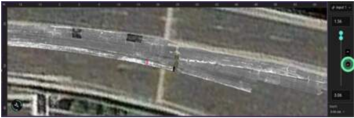
Figure 5. Major surface defects at asphalt layer (cracks)
