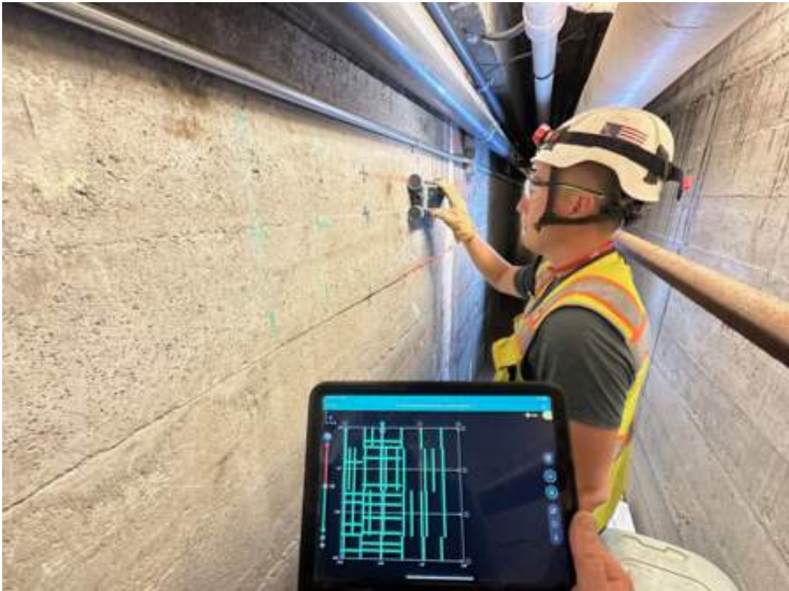
Reinforcement detailing with the Profometer PM8000 Pro cover meter, visualizing the results instantly on the iPad
