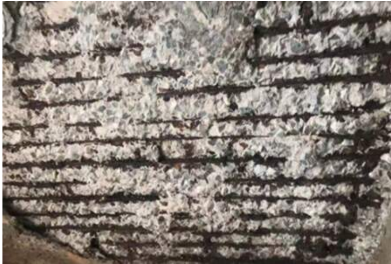
Rusting and peeling areas (front plate)
