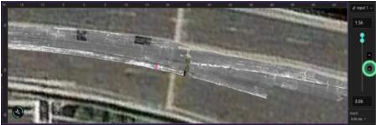
Figure 5. Major surface defects at asphalt layer (cracks)
