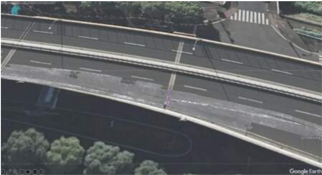
Figure 1. C-scan view overlaid in Google Earth, depicting the analysis of surface defects obtained from GPR Insights data collected by the GS9000.
