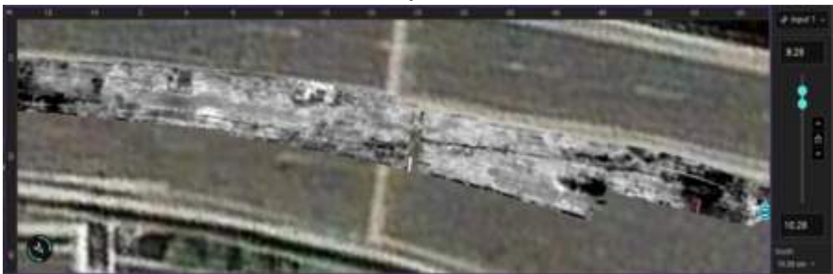
Figure 7. Interface defects between Asphalt-to-Concrete (A/C) layers (Delamination.)
