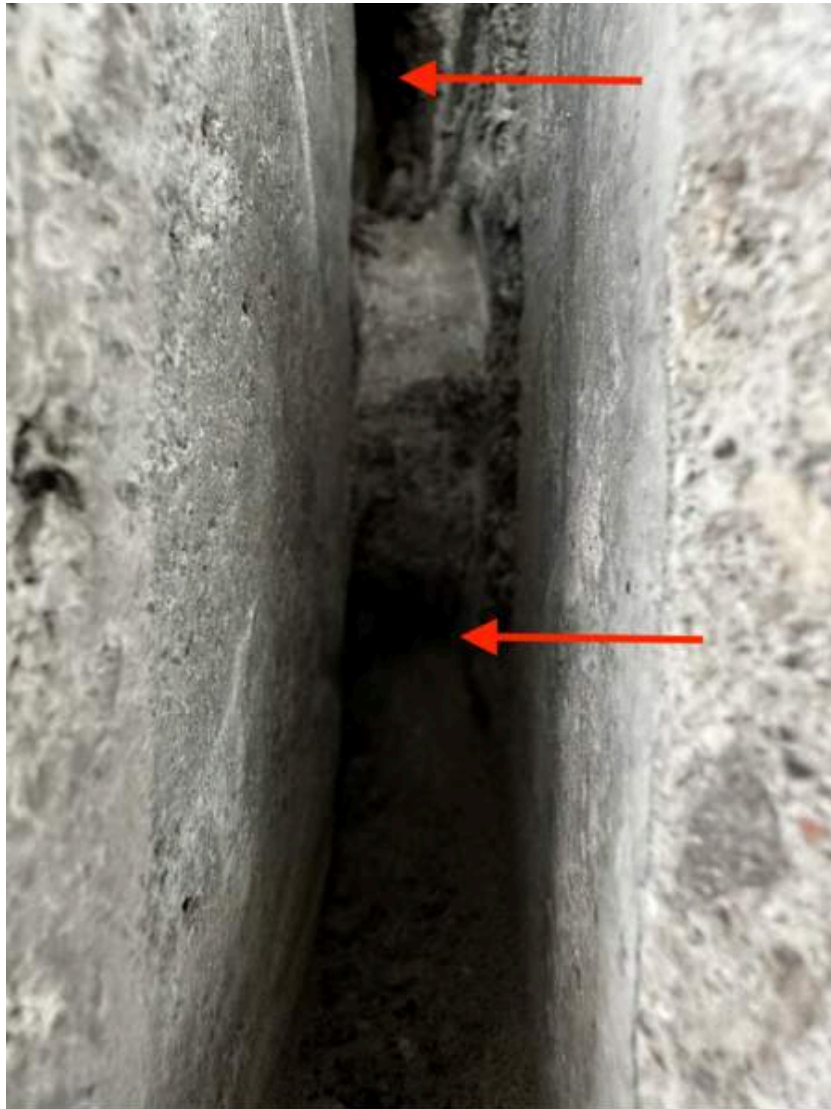
located voids in the joint
