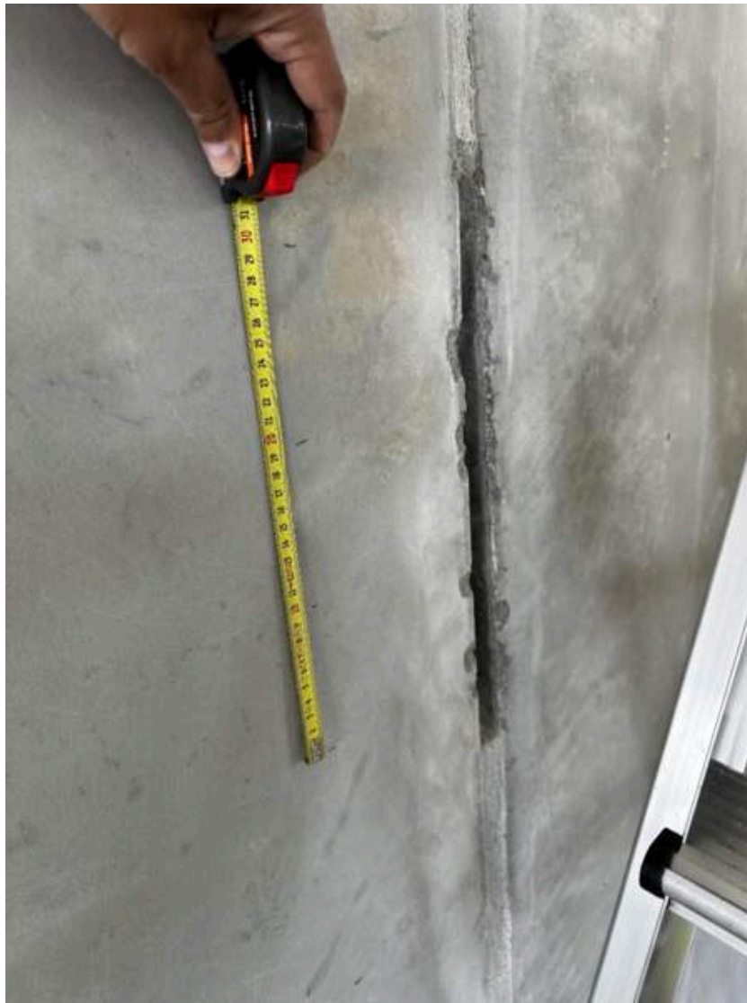
Voiding found over a 30cm length (they didn't break out the entire length of the void. Total length of voided joint section was estimated at 45cm)
