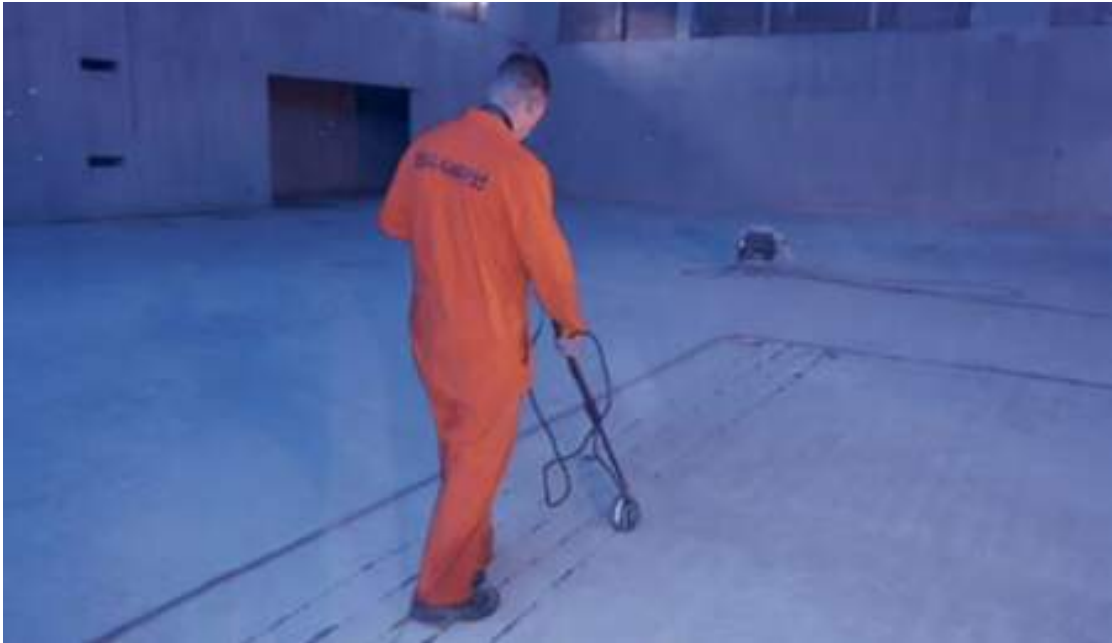
Performing half-cell potential measurements on the concrete floor with the Profometer PM8500 corrosion sensor
