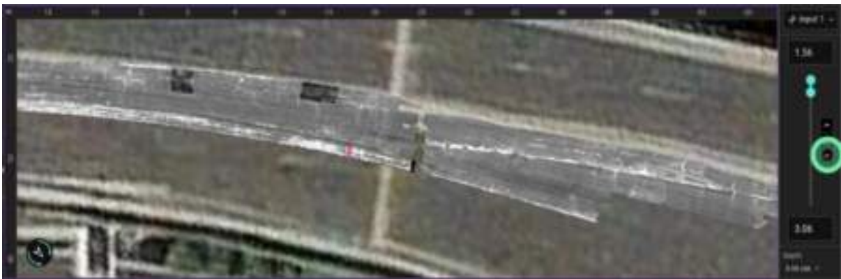
Figure 5. Major surface defects at asphalt layer (cracks)
