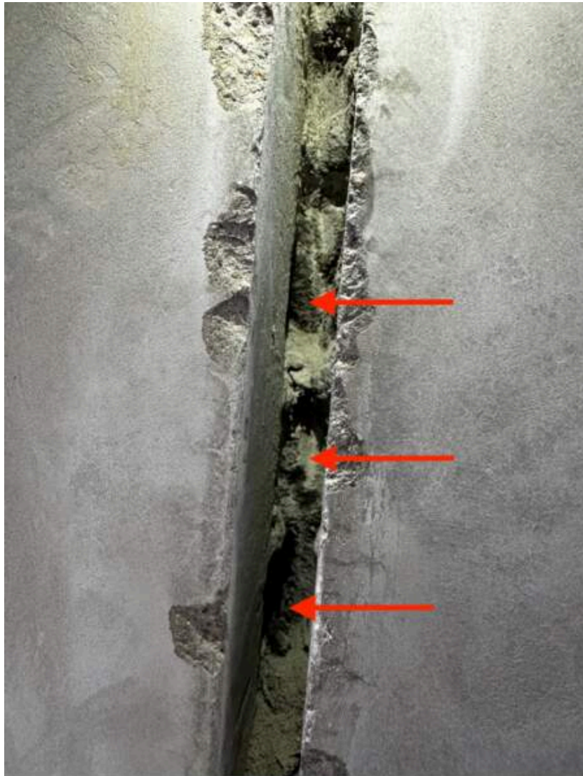
First scan location was voided in joint where red arrows are
