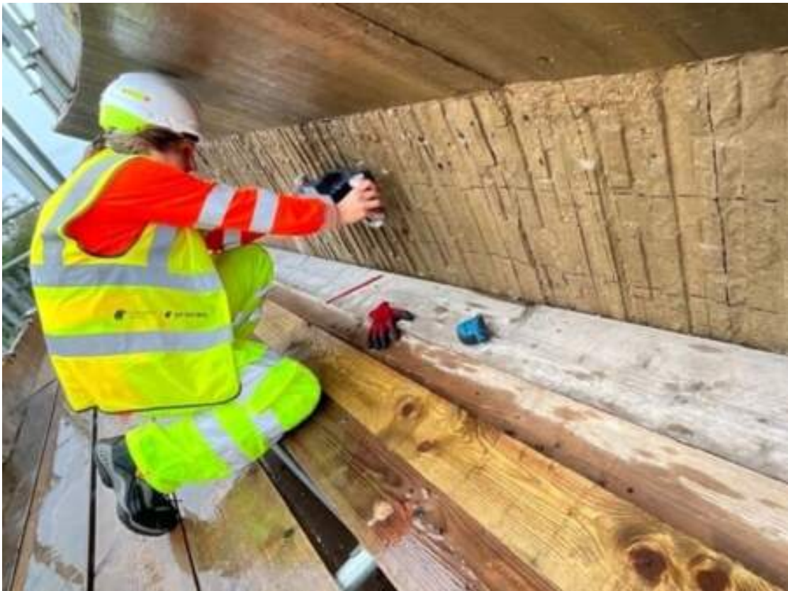
The Pundit PD8050 being used to detect hidden voids in the concrete.
