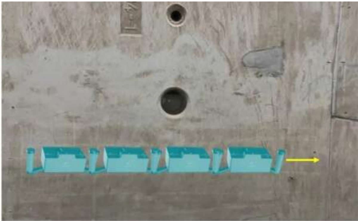
Scanning in the direction of the yellow arrow with ultrasonic imaging
