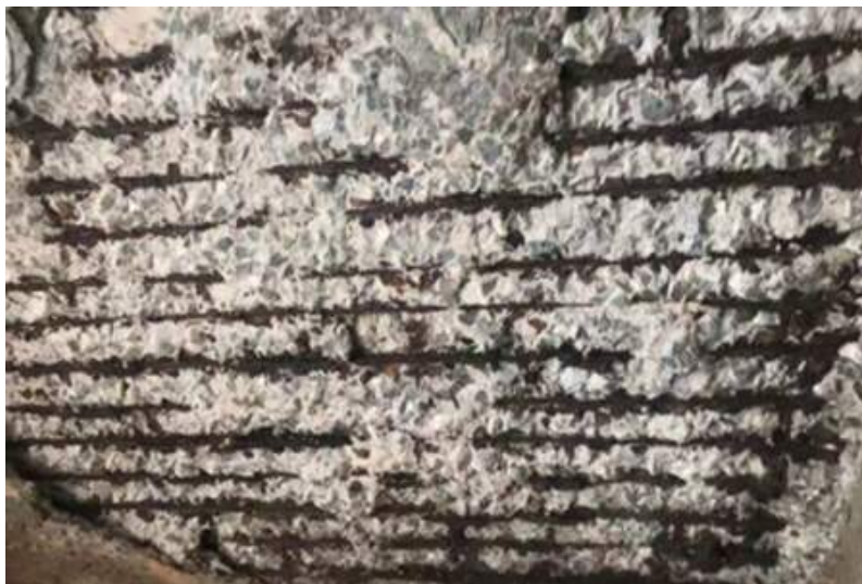
Rusting and peeling areas (front plate)
