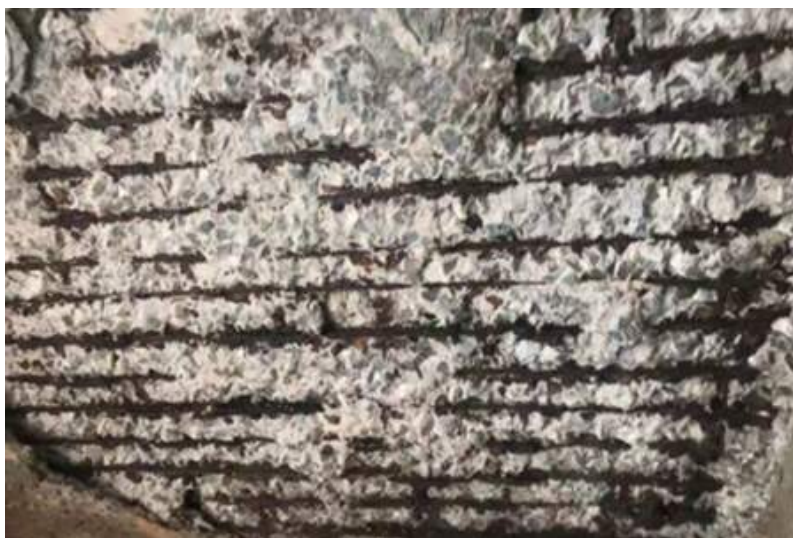
Rusting and peeling areas (front plate)
