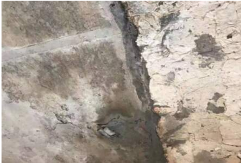
Undamaged areas (back plate)
